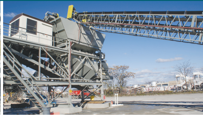
Left: Construction of Taxiway KC. A major portion of the reconstruction project will be done without interruption to service.
